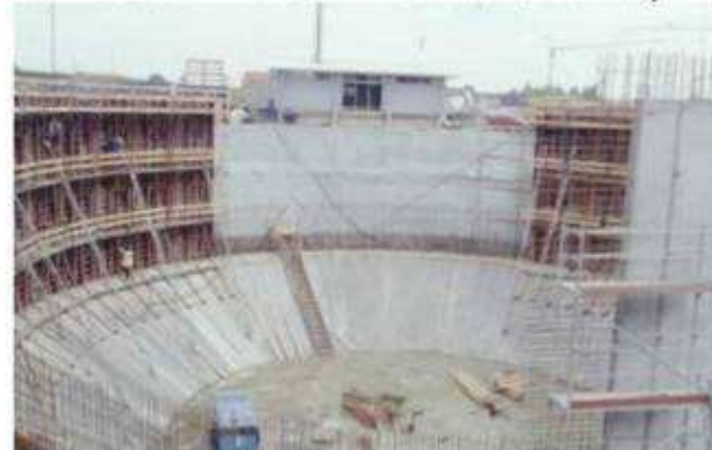
12,000 m 3 seasonal storage, Friedrichshafen, Germany
